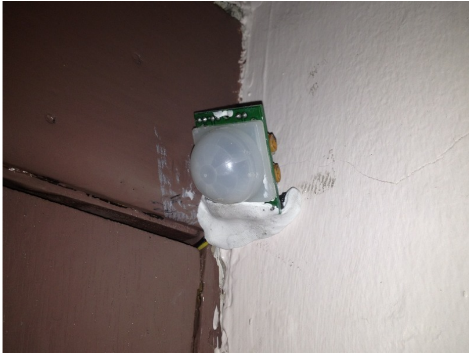
Mounted PIR sensor with some Sugru (http://adafru.it/436)
