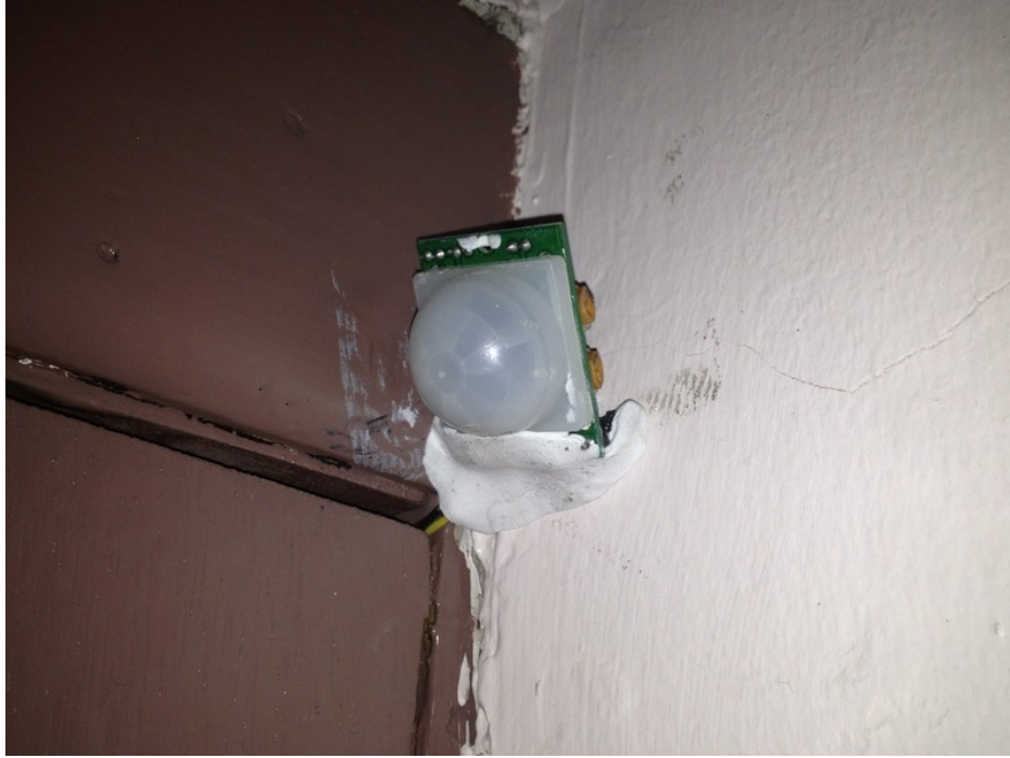
Mounted PIR sensor with some Sugru (http://adafru.it/436)
